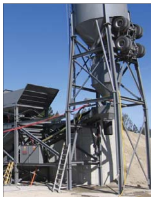
Concrete portable plant
